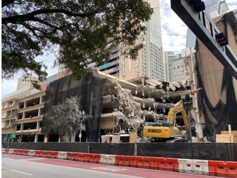
Figure 10: Demolition of the former First National Bank building on December 21, 2024. Courtesy of Casey M. Picket.
